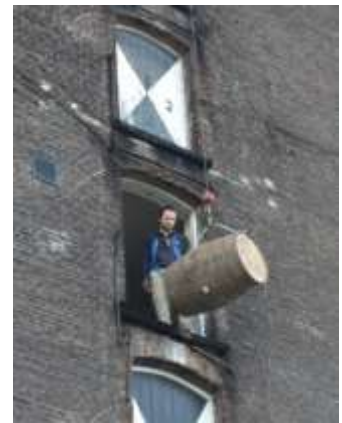
Brewery buildings and a hazardous operation at Het Anker
